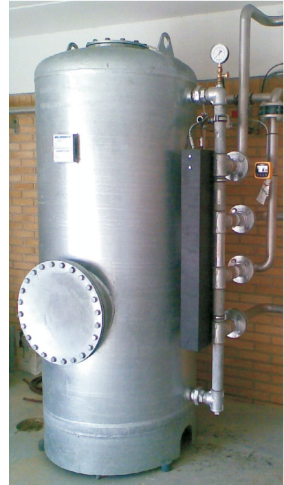
Arsenic removal by means of adsorption in waterworks. The solution comprises an automatic pressure filter type NSB 170 installed after open filters. Flow rate: 12 m 3 /h.
