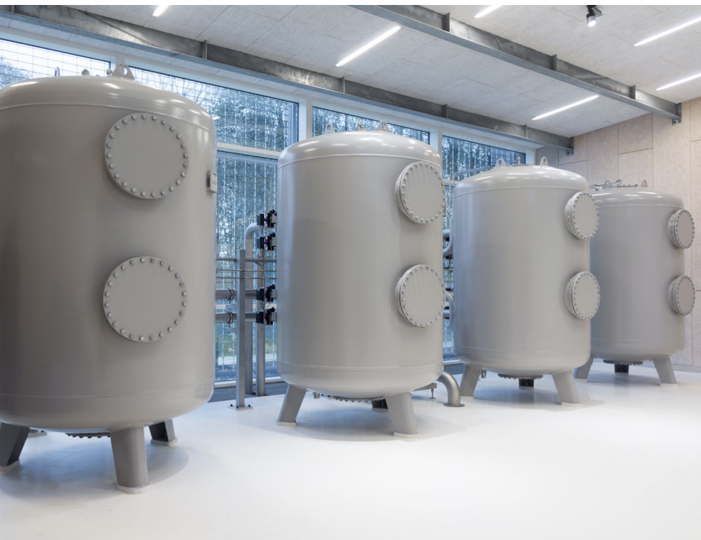
Removal of iron, manganese, and ammonium in waterworks. Flow rate: 2 x 30 m 3 /h.
