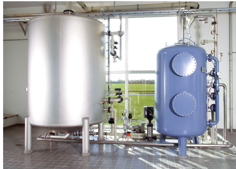
Degassing of dissolved gases such as aggressive carbon dioxide, methane, and hydrogen sulphide is a precondition of optimum filtration. Photo: degassing and pressure filtration in brewery.
