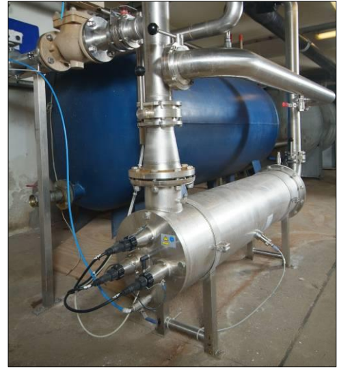
UV system type Spektron 70 with a flow rate of 108 m 3 /h. The system is installed in a dairy.
